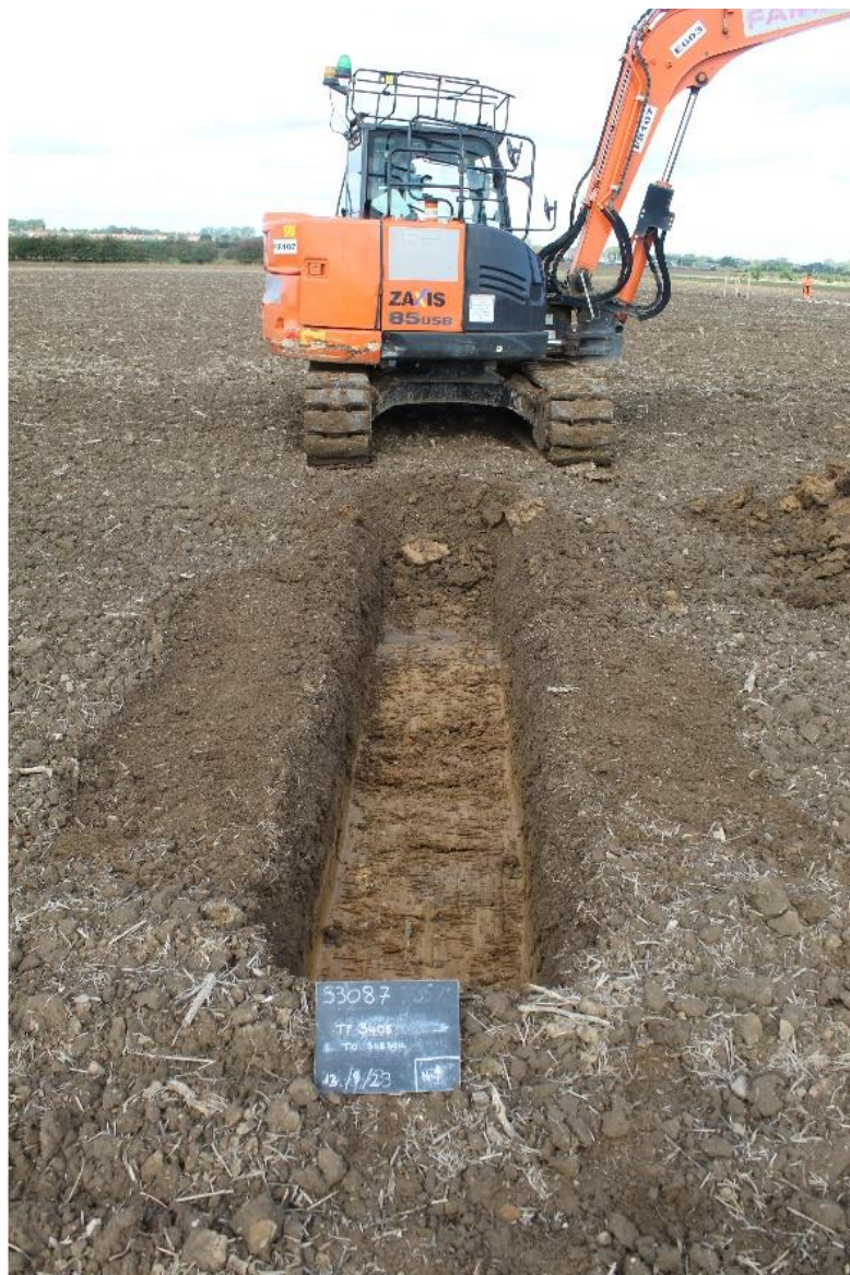
Plate 5: Test pit [3405] excavated to the top of the subsoil, viewed from the south.
